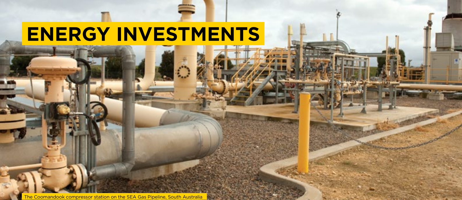
The Coomandook compressor station on the SEA Gas Pipeline, South Australia
